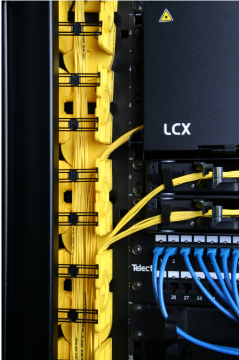
Figure 3: Close-up of cable entrance and exit points in a flexible link cable management system
