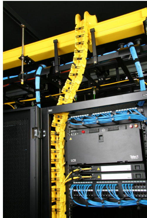
Figure 2: Using flexible links for an overhead drop in a datacenter Note the curve of the drop
